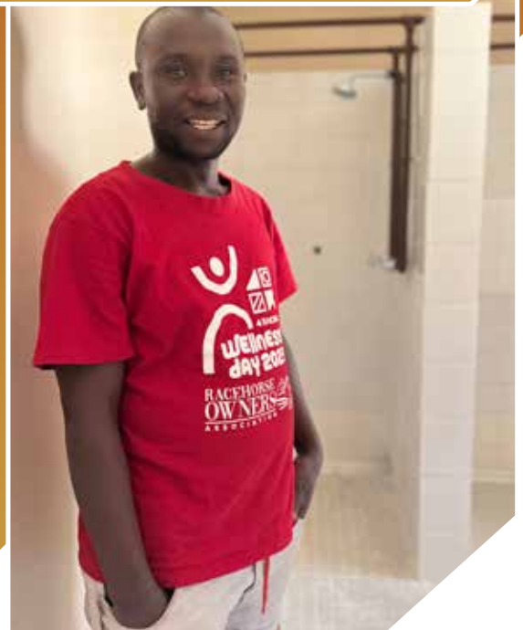
Grooms from the Fabian Habib stable, Moses Zhuwau (red shirt) and Buti Makoe showcase the progress being made with the renovation of the grooms accommodation at Turffontein Racecourse
